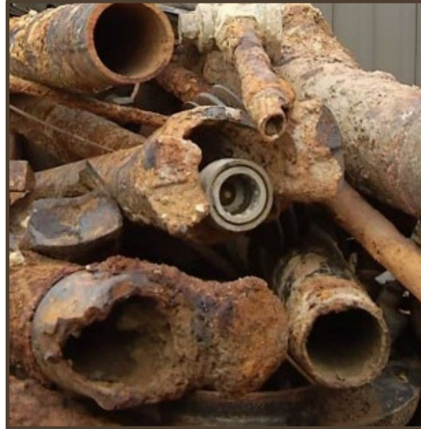
Human-caused contaminants from plumbing (Lead & Copper)
